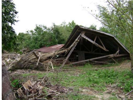
A collapsed primary school
